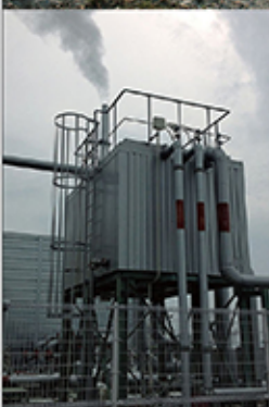
Obama Binary Power Plant
